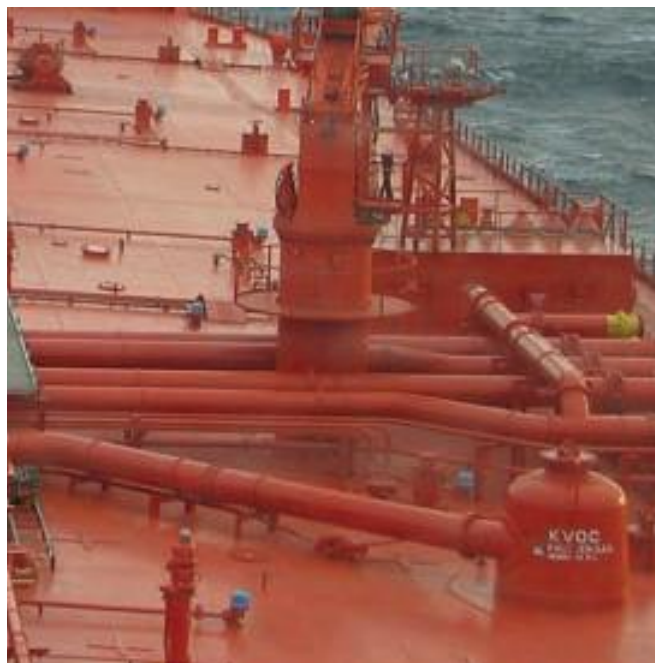
KVOC® drop pipe installed on Sallie Knutsen
